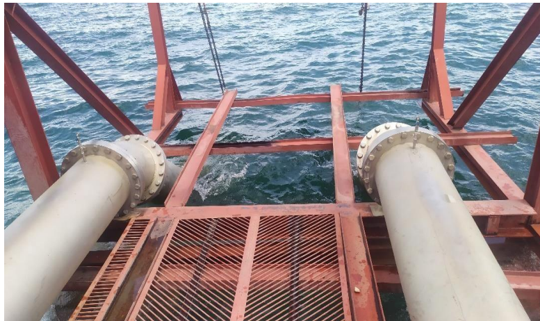
Figure 2-1. Station de captage Lac II [26]
