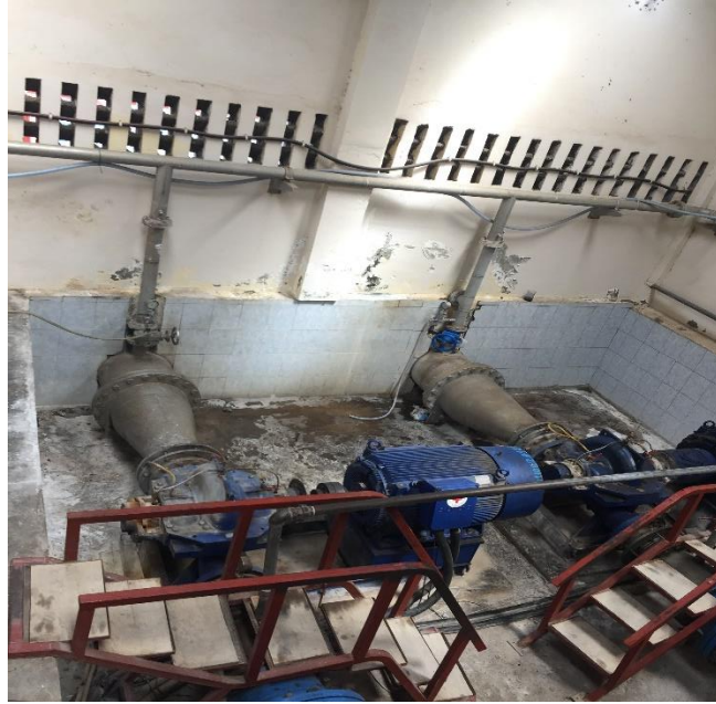
Figure 2-2. Salle des machines [26]
